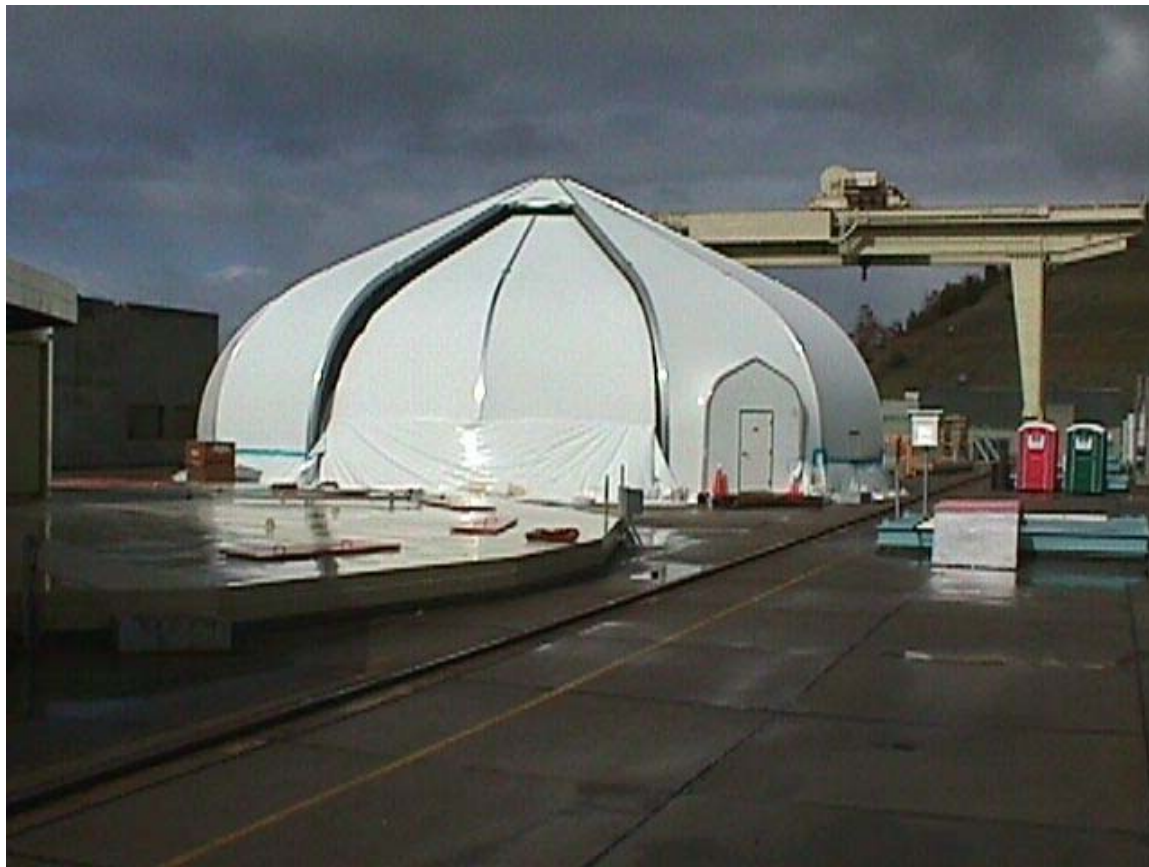
Figure 1. Exposed generator with weatherproof enclosure
