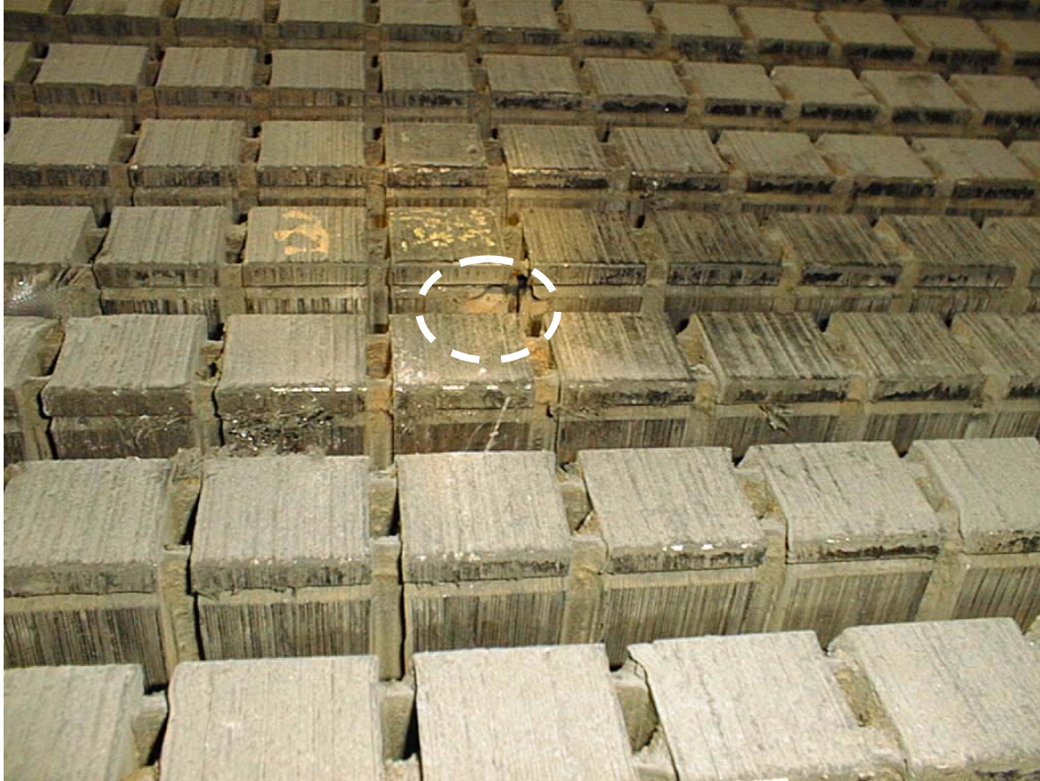
Figure 18. Visual Confirmation of Damaged Area
