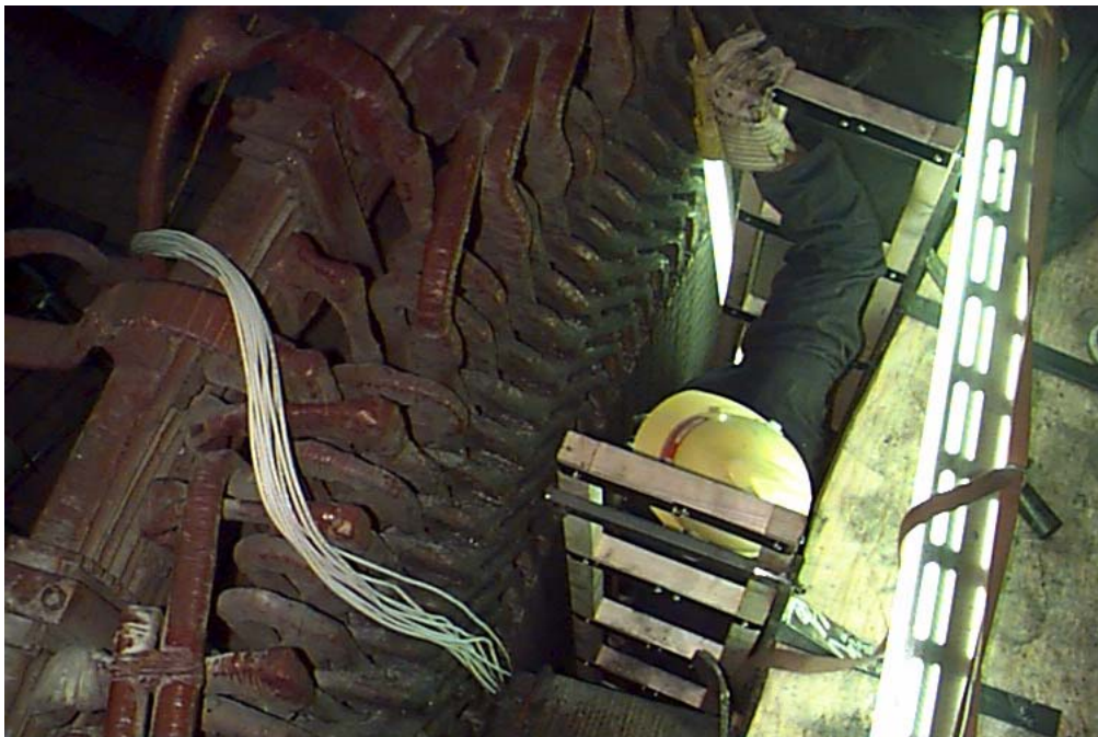
Figure 8. One of four bundles of excitation cable (7 turns)
