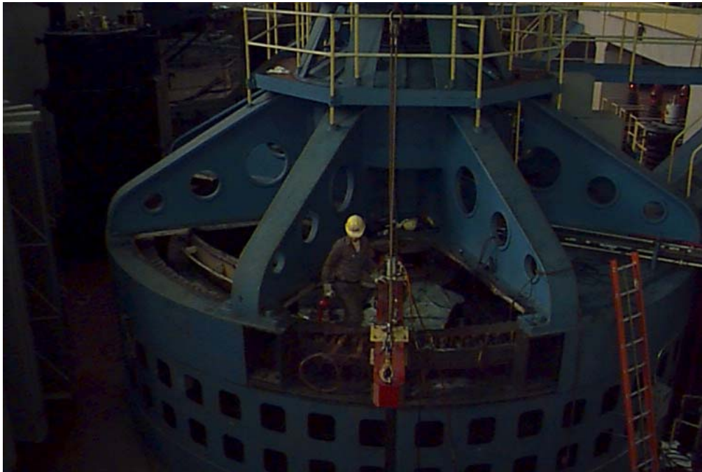
Figure 6. Unit #4 at ALCAN's Chute a Caron facility
